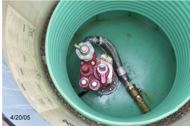
Showing a mechanical line leak detector
