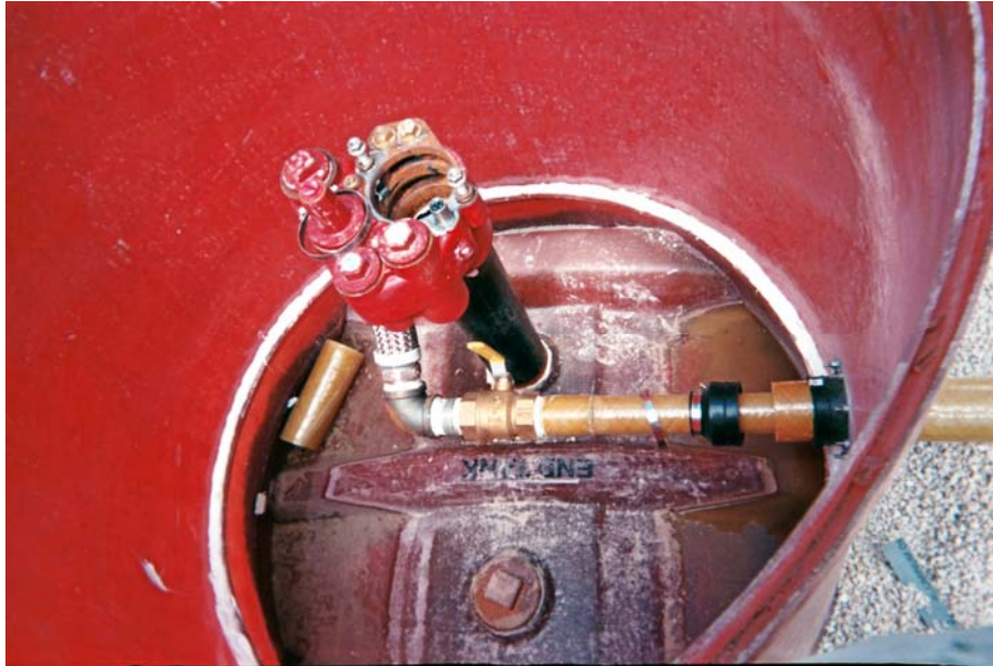
This photo shows double-wall FRP piping
