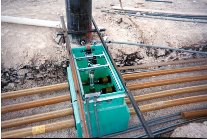
Dispenser sump with emergency shut-off valve
