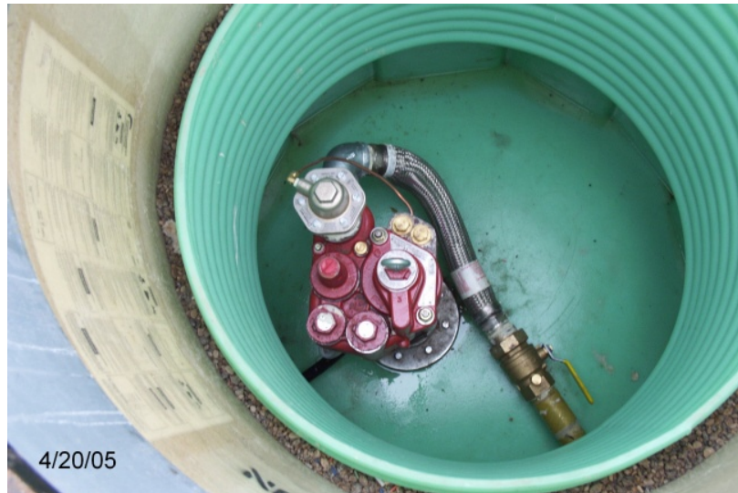
Showing STP to supply fuel to the dispensers
