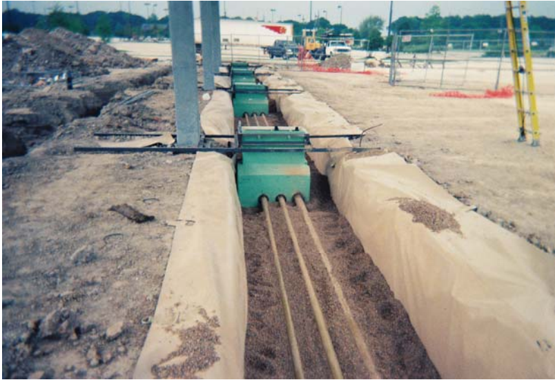
Showing sumps at the dispenser islands
