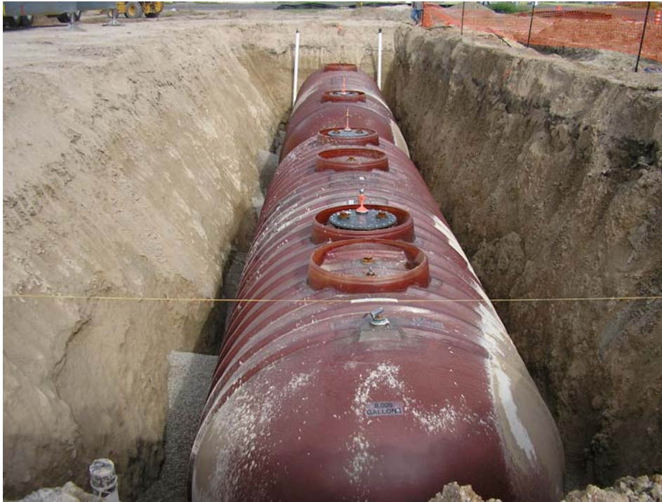
Showing a different make of FRP tank
