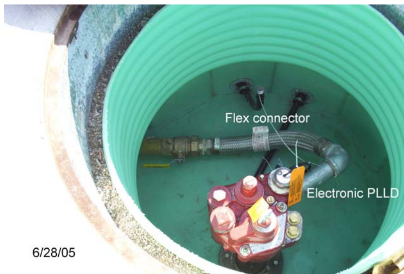
Showing an electronic line leak detector and flexible connector
