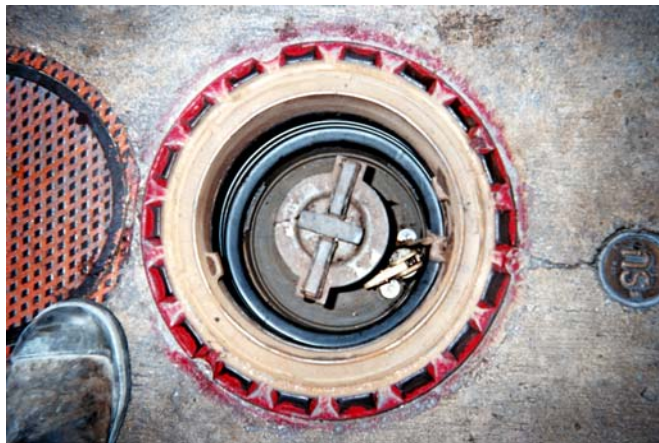
Showing a 5-gallon spill containment bucket on the fill tube
