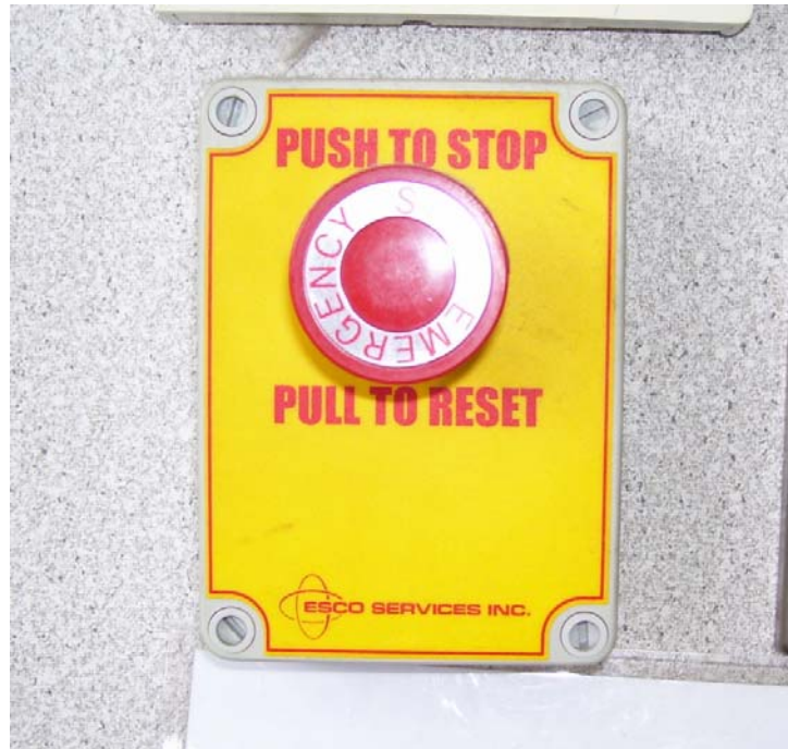
Emergency stop, this one located inside the store.
